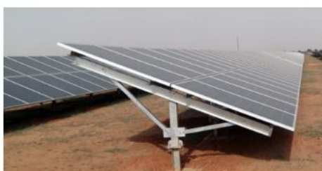
Seasonal Tilt Solar Structure
